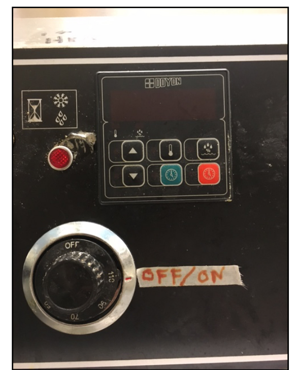
Figure 10. Doyon bread proofer w/ electrical control panel re-wired to oven dial controls after maintenance repair.
